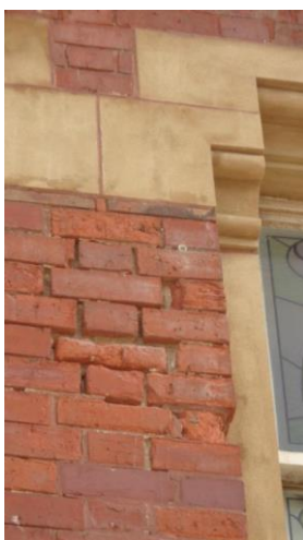
Spalling Victorian brickwork pointed with cement mortar
