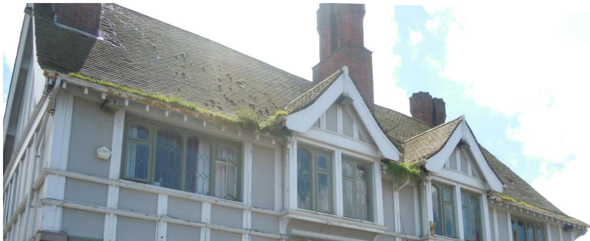
Gutters which need to be cleared of vegetation to prevent water ingress
